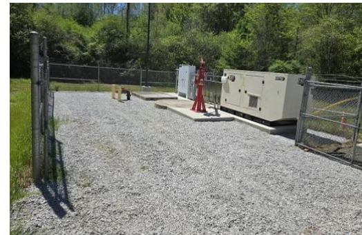
Freeman Creek Lift Station
